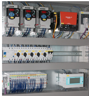
Full SPS integration for training under real conditions
